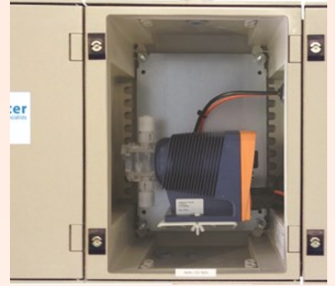
Tamper Proof Cabinets
